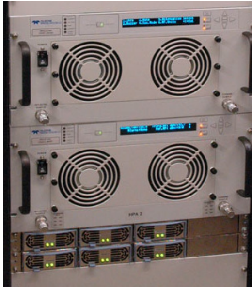
C-Band 1:1 Redundant System in the 5RU chassis, with N+1 redundant power supplies
